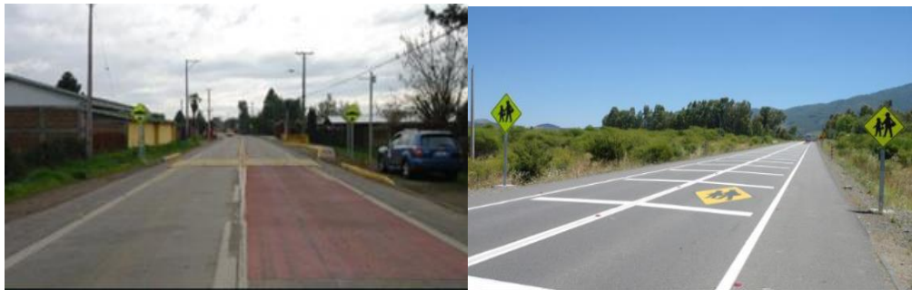
Figure 3: Speed hump (left), Transverse lines on both lanes (right) (Source: PIARC, 2019)
